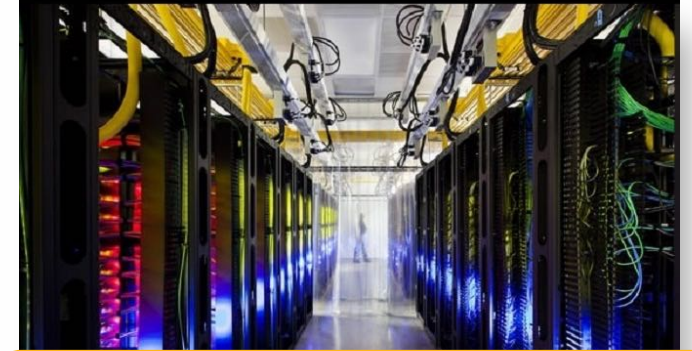
Cloud Infrastructure Multi-Gbps networking
